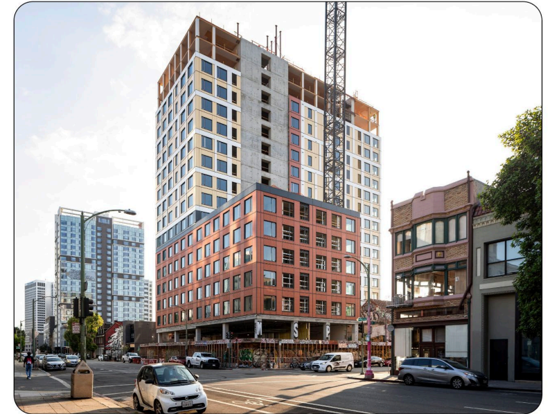
oWow, a winner of StopWaste's Environmental Leadership Award for Excellence in Construction Innovation.
